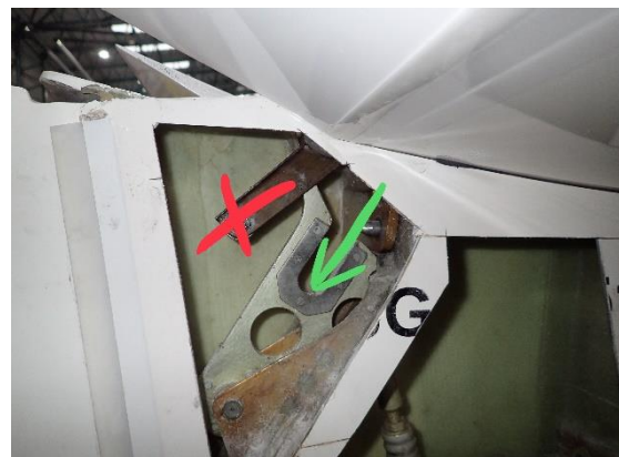
Disconnected elevator control
